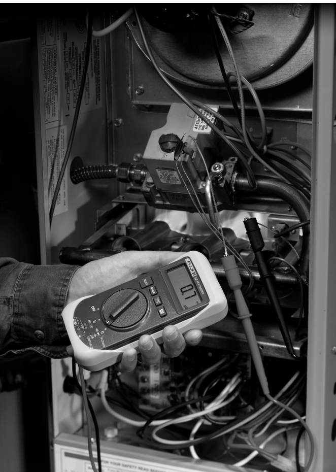
Figure 19. Fluke 16 in the microamps mode testing the flame rod rectification circuit.
