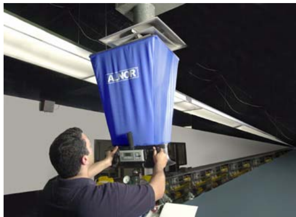
Electronic Balometer measuring a supply diffuser
