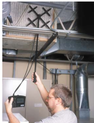
Velocity matrix measuring face velocity of an HVAC filter
