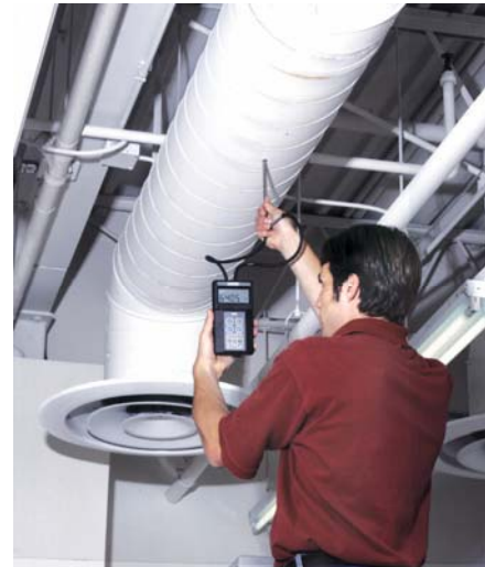
Duct traverse with AXD560 Micromanometer and pitot tube
