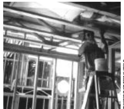
The effects of duct leakage on cooling loads, which have only recently come under scrutiny, are not included in any of the methods mentioned here. However, any leakage will naturally impact the overall HVAC system. Here, a worker seals the ducts before the drywall is installed, while all the joints are still easily accessible.
